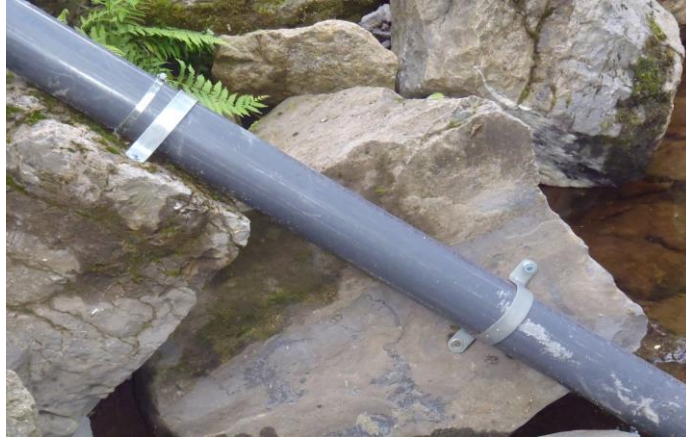
Figure 1. Instream Sonde Installation
