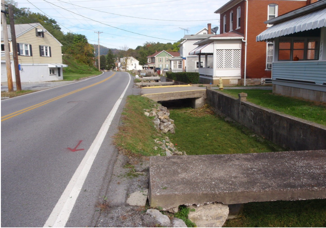
Figure 7-7. Cabbage Creek Flowing under the Driveways of Homes in Roaring Spring (The plant growth in the stream is predominantly watercress.)
