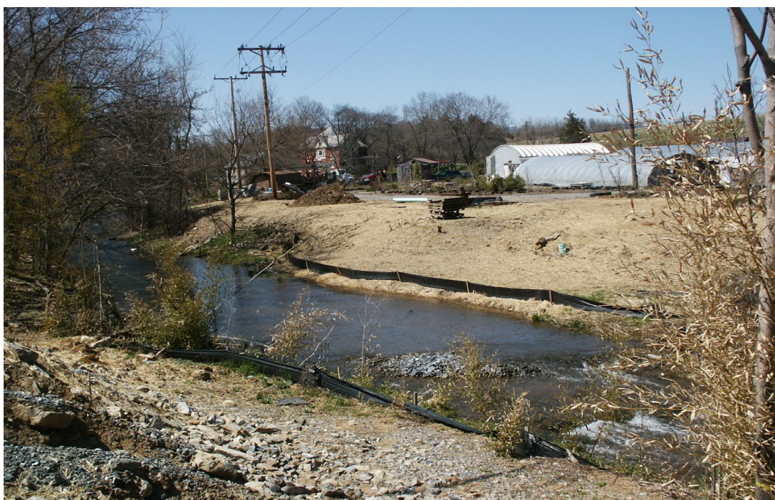
Figure 7-14. Siltation Fencing and Constructed Banks along a Reach of Three Springs Run
