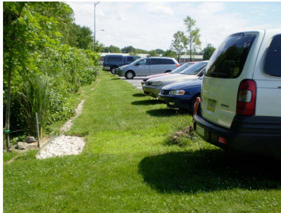
HACC Underground Infiltration Unit
