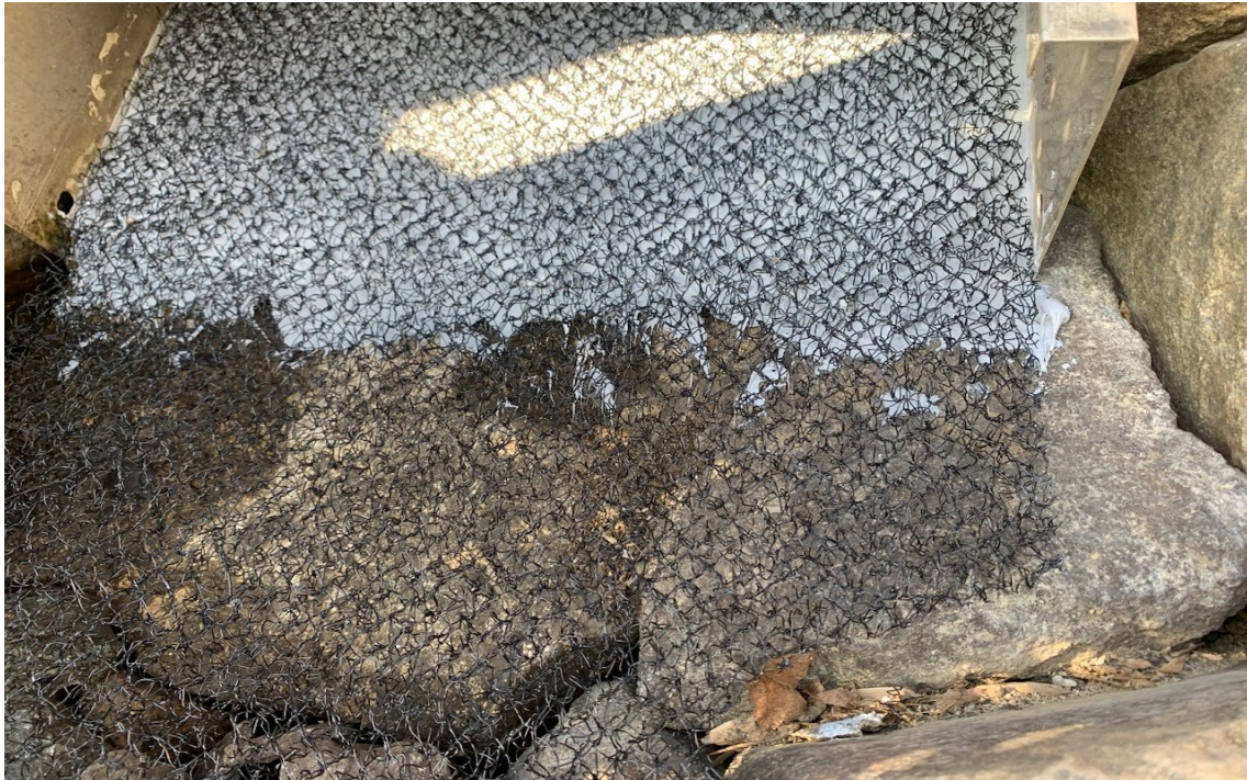
Figure 5.0-1: Transition from Riprap Shoreline to Ramp Entrance, Conowingo West Eel Collection Facility, 2022
