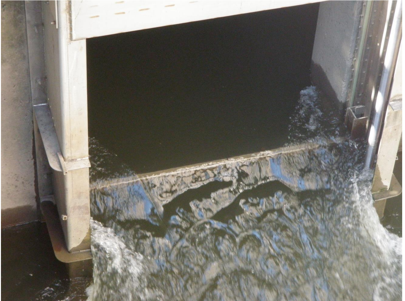
Figure 1: Gate C steel bar crossing through the water column, right at the path that fish would use to move into the fishway
