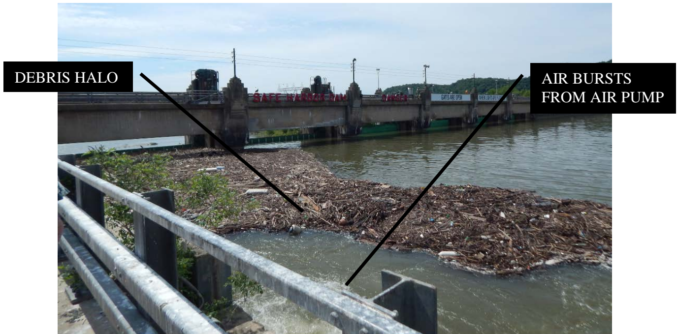
Figure 1 – Debris accumulation in the vicinity of the exit channel trash rack
